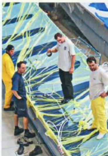
Vacuum-infusion technique: the epoxy resin is spread evenly over the fibres using vacuum pressure.
